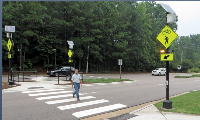
Crosswalk w/Solar Powered Rectangular Rapid Flashing Beacon
